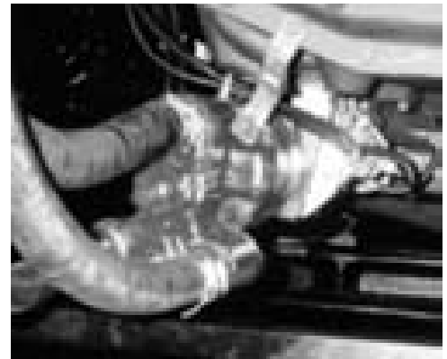
Improper Bracket Installation
